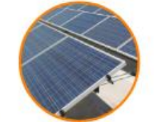
Rooftop Solar PV System
